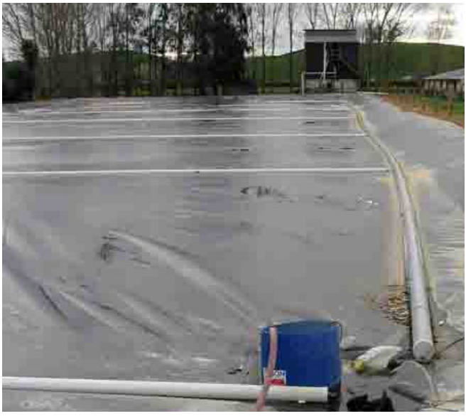
Covered Anaerobic Pond showing layout of weight pipes and rainwater pump
